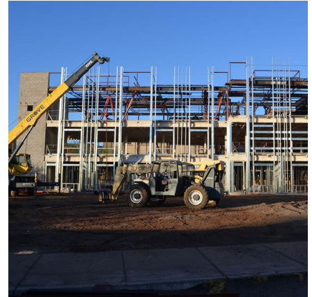
During construction of a new phase at Sagewood, Weitz developed a temporary access drive for the CCRC that ensured full access to the community and enabled the new entrance to Sagewood was delivered earlier than expected.
