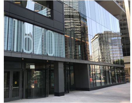
Collaboration with the design team contributed to successfully renovating this four-story podium and amenities area without adversely affecting the building's 3,000 occupants.
